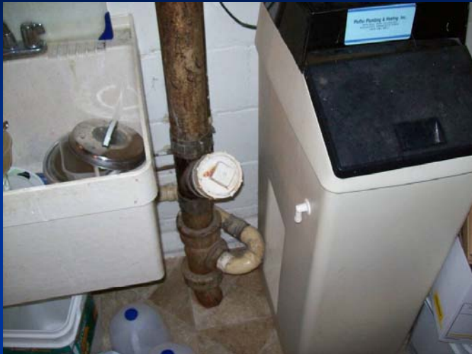
Illicit Sump Connection
