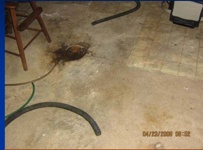
Illicit Sump/Hose Connection
