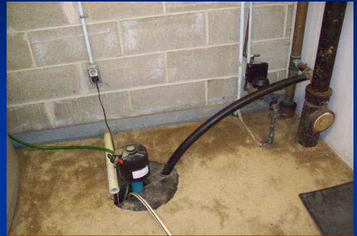
Illicit Sump Connection
