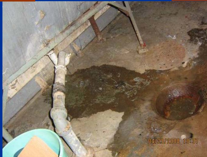
Artificial Seepage Collection System (Beaver Drain)
