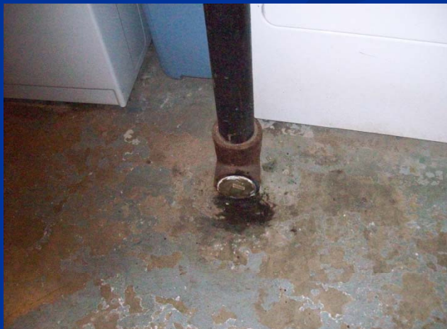
Inaccessible – Clean Out In Concrete
