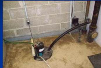
Illicit Sump Connection
