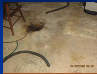
Illicit Sump/Hose Connection
