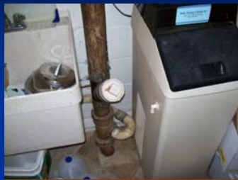
Illicit Sump Connection
