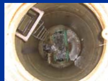
Leaking Pipe Seal
